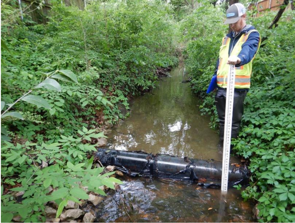
Station 4+50 - Looking upstream, this photo shows the exposed sewer line at this location and illustrates the concern with Area of Concern #3 .
