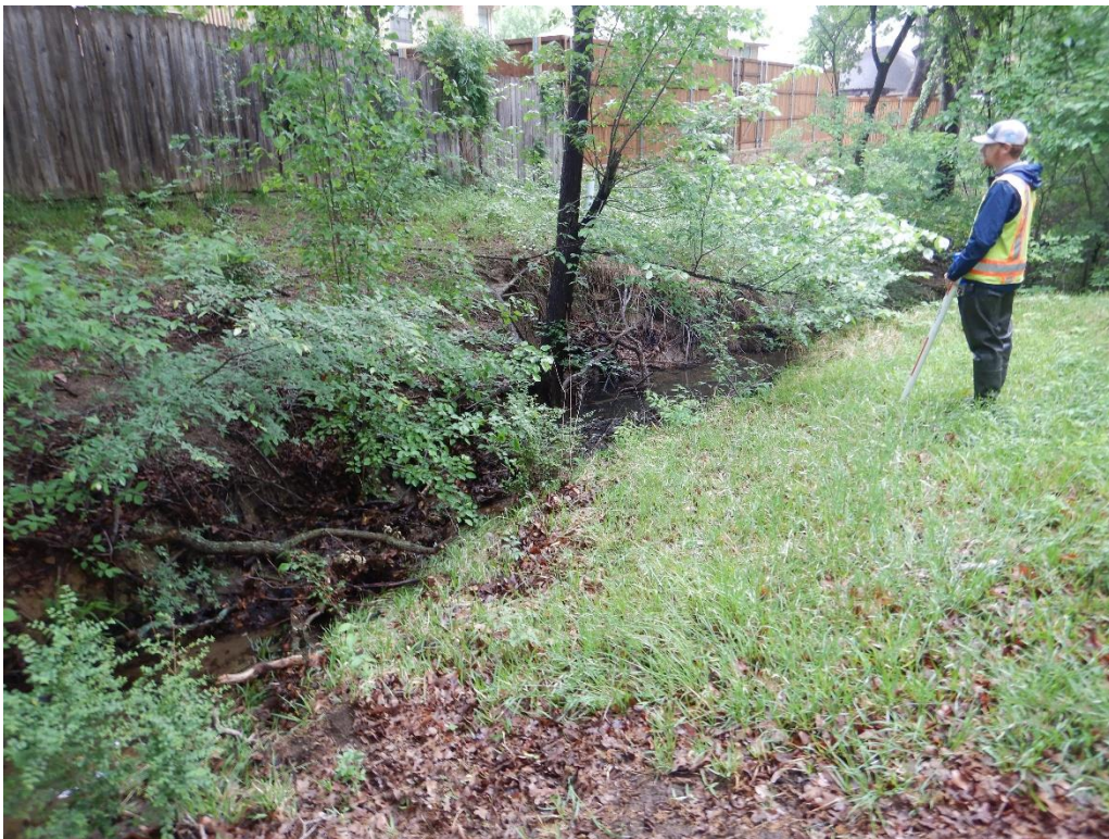
Station 3+25 - Looking at left bank, this photo shows representative conditions, including isolated bank erosion near home backyards. This photo illustrates the concern with Area of Concern #2 .
