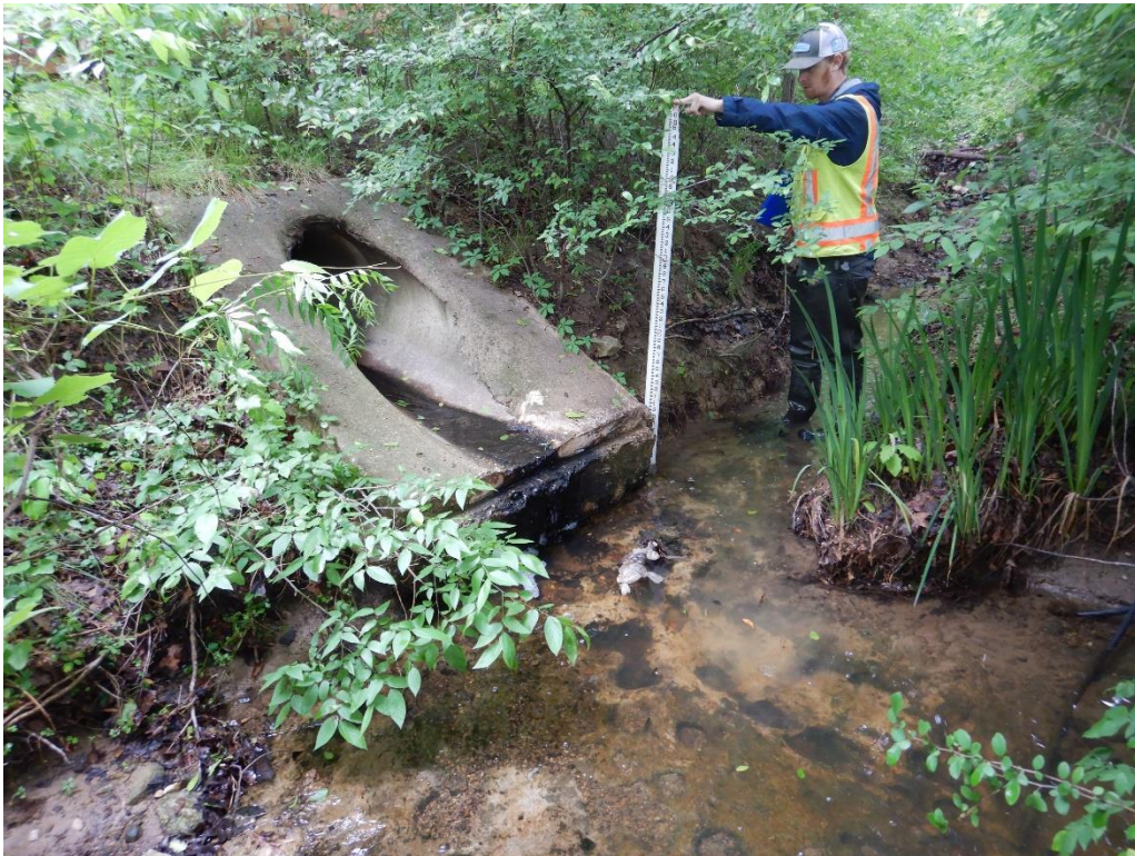
Station 5+75 - Looking upstream at the right stream bank, this photo shows the condition of the stormwater outfall and the beginning stages of downcutting at scour ( Area of Concern #4 ).
