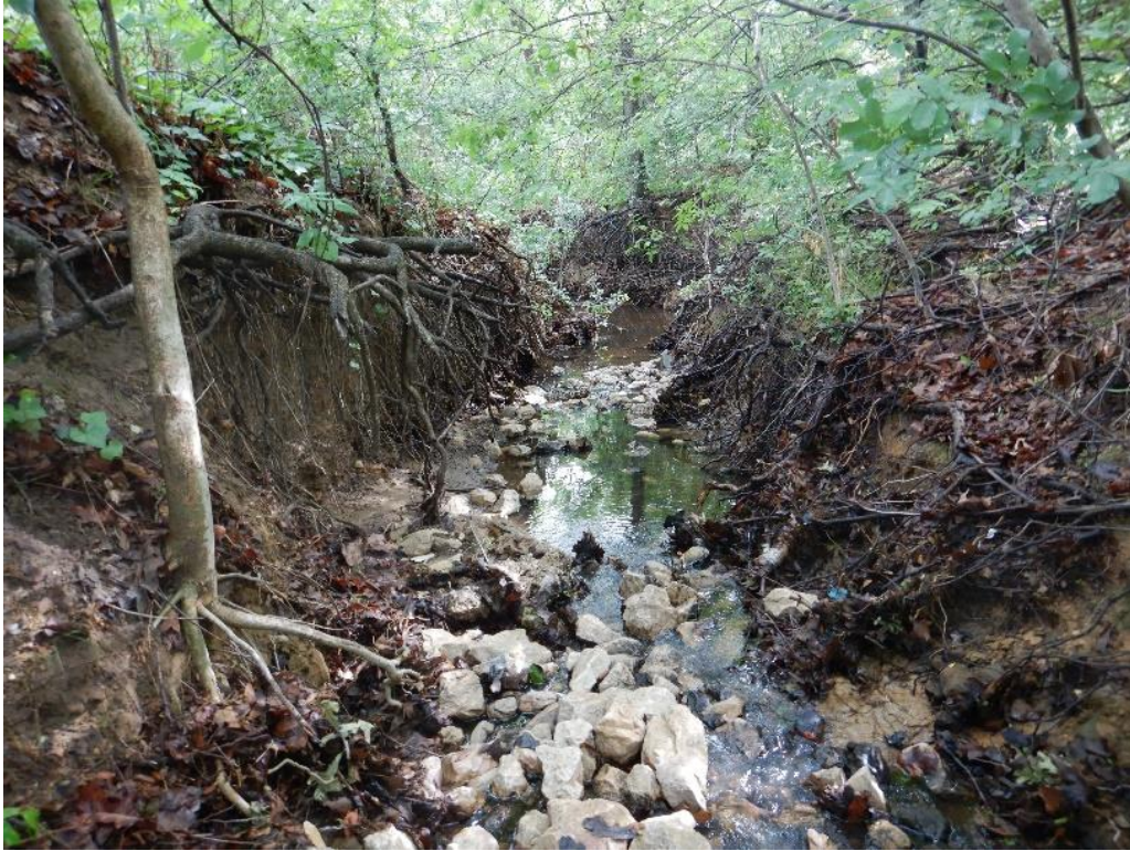
Station 8+50 - Looking downstream from the exposed sewer line showing the scour and bank erosion adjacent to Area of Concern #7 .
