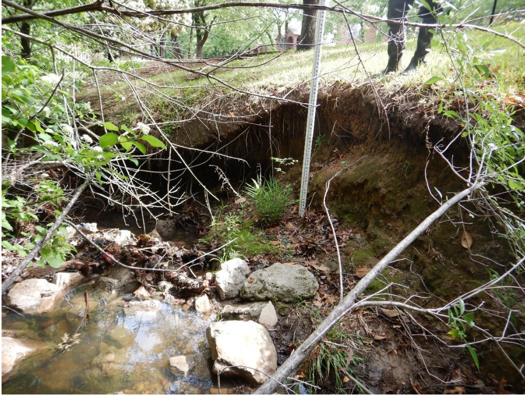
Station 14+90 - Looking at right bank, this photo shows the bank undercutting immediately upstream of the grouted rip rap protection of Creekside Ct ( Area of Concern #10 ).
