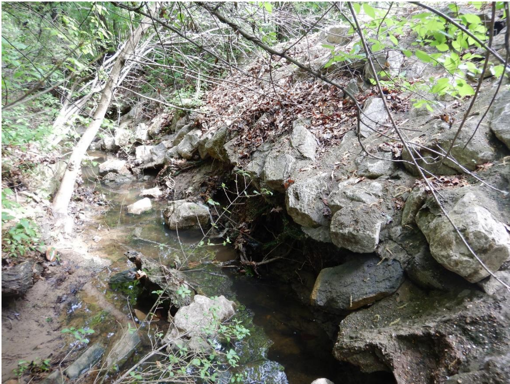
Station 15+15 - Looking downstream, this photo shows the undercutting below bank protection measures at this location ( Area of Concern #10 ).
