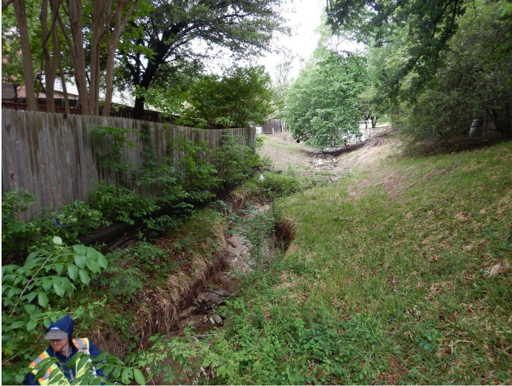
Station 1+00 - Looking upstream the beginning stages of downcutting and headcut migration can be observed. This photo shows Area of Concern #1 .
