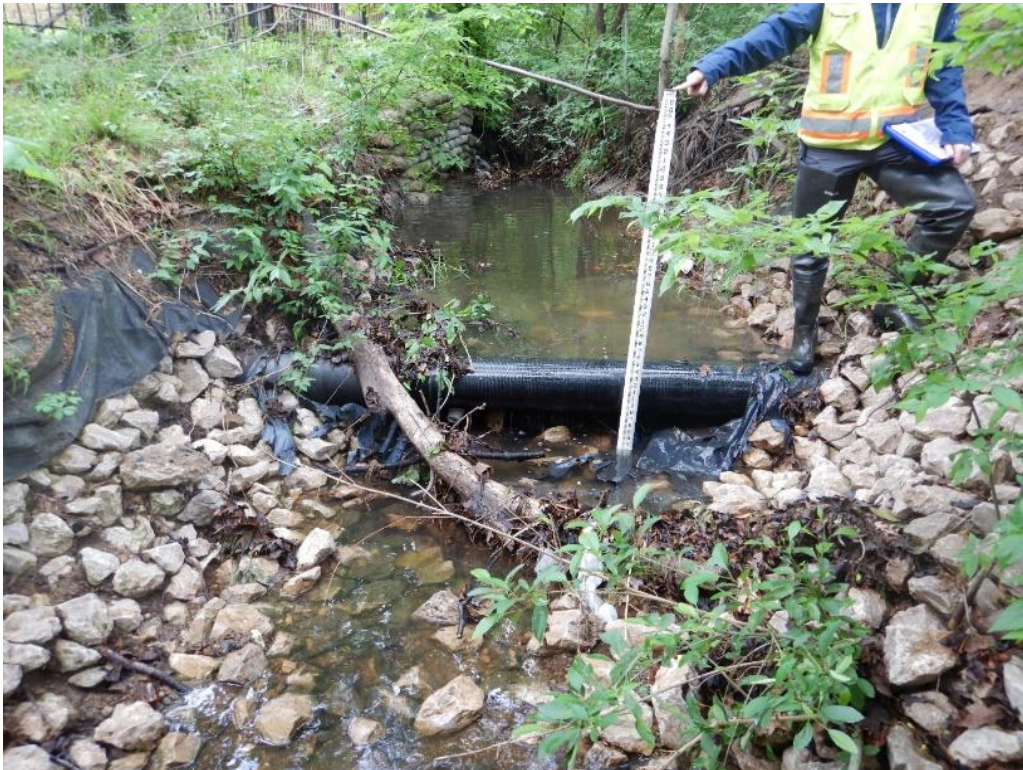
Station 8+50 - Looking upstream at the location of an exposed sewer line ( Area of Concern #7 ). This photo shows how the sewer line is holding the grade of the stream.
