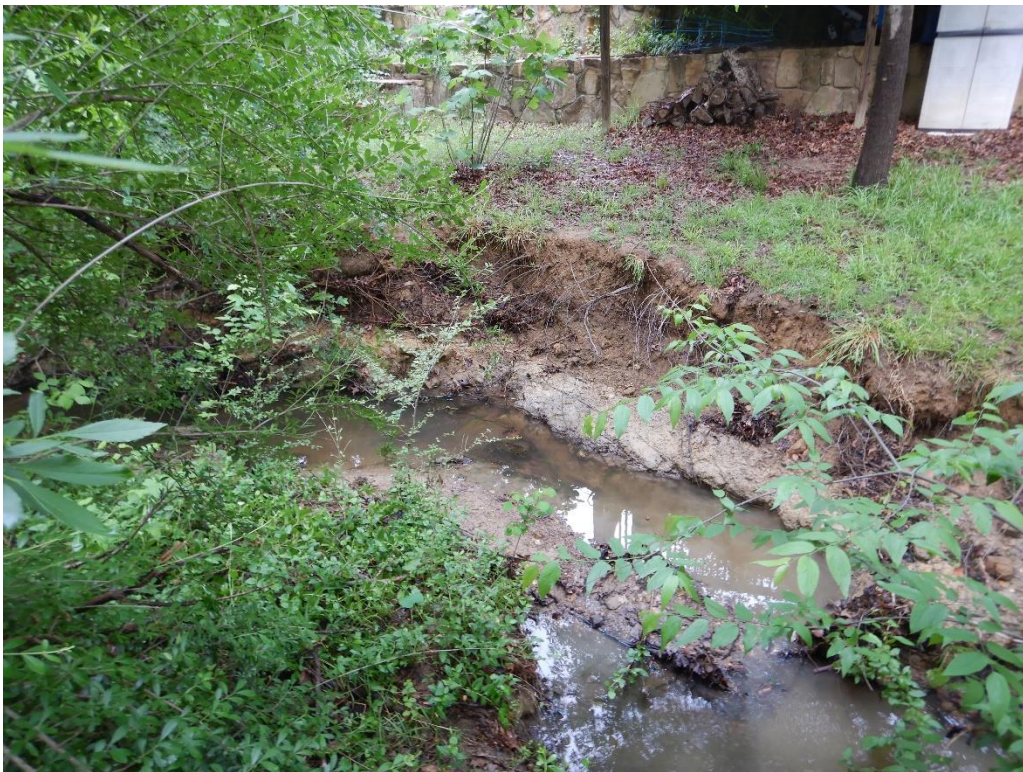
Station 11+25 - Looking at the left stream bank, this photo shows the bank erosion below the headcut and impacts to a nearby property ( Area of Concern #8 ).
