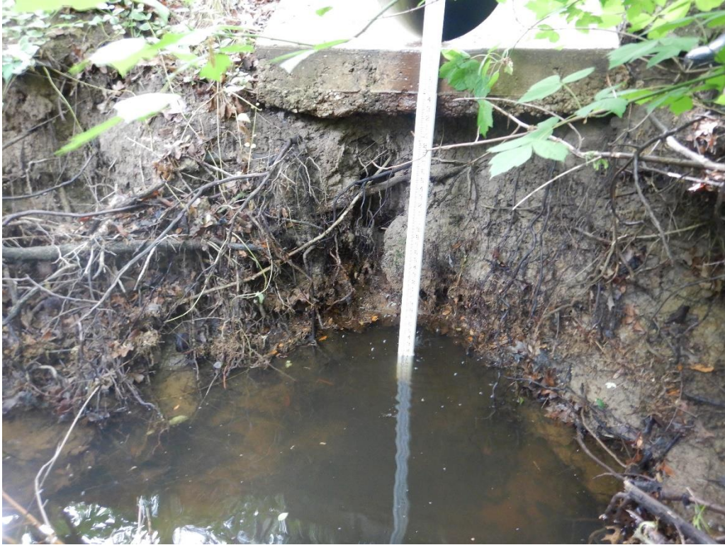
Station 7+75 - Looking at the stormwater outfall on the right stream bank, this photo shows scour beneath this structure ( Area of Concern #6 ). Bank scour of similar magnitude is occurring on opposite bank.
