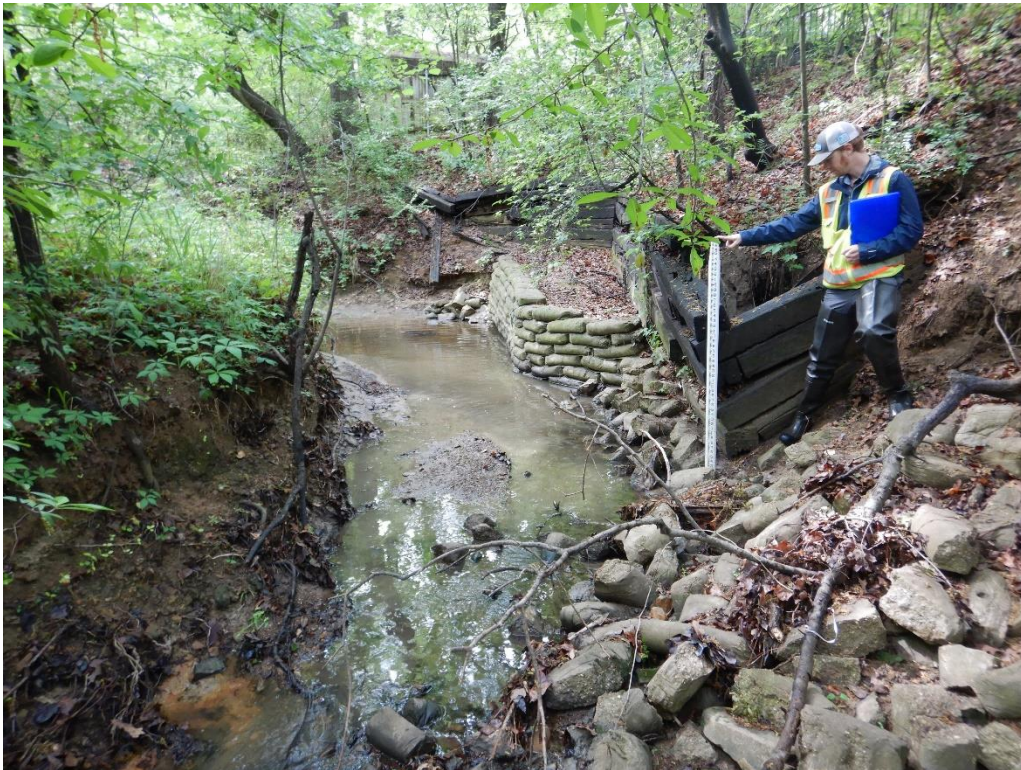
Station 17+50 - Looking upstream, this photo shows the failing bag wall and railroad tie wall behind a home ( Area of Concern #12 )
