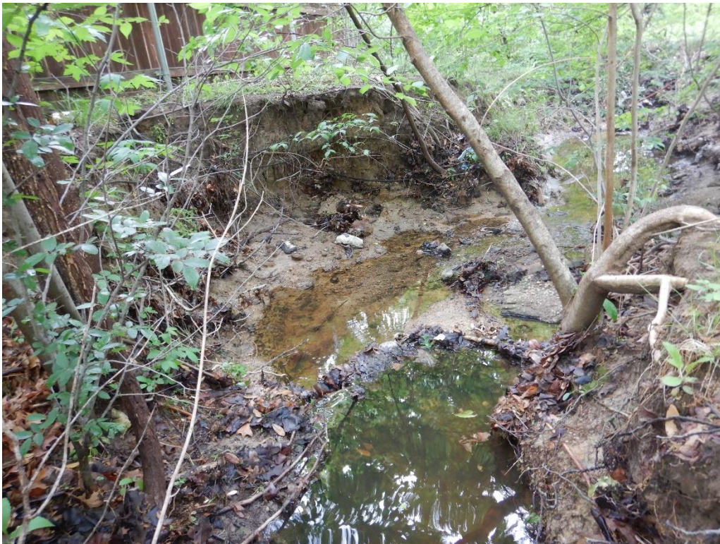
Station 7+00 - Looking downstream, this photo shows representative conditions and bank erosion into home backyards (Area of Concern #5)
